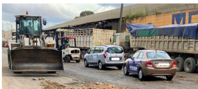
Figure 23: Pothole repairs, Abidjan. Source: CITAC.
