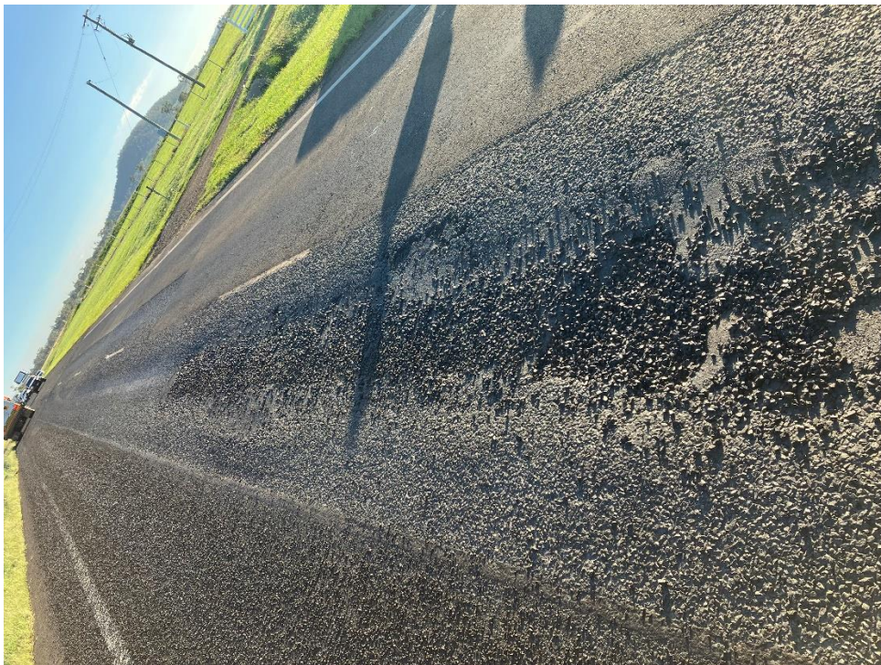
Figure 3, Existing Failures example
